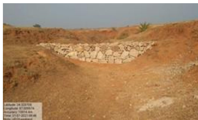
Loose Boulder Structer
